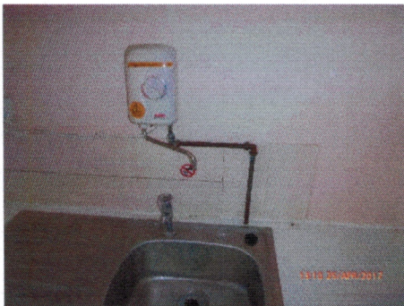
Photo 9: Broken water heater in Vickers 1st floor Kitchen
