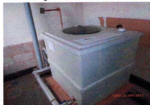
Photo 6: CWST 3 in Vickers House with 1 redundant outlet feeding a decommissioned calorifier
