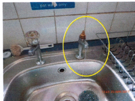
Photo 12: Example of faulty outlets in the canteen
