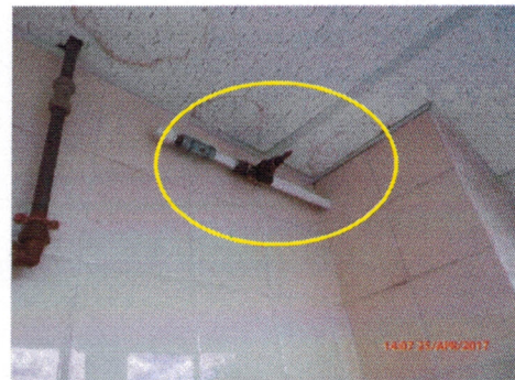
Photo 16: Deadend in Century house 1st floor male toilet
