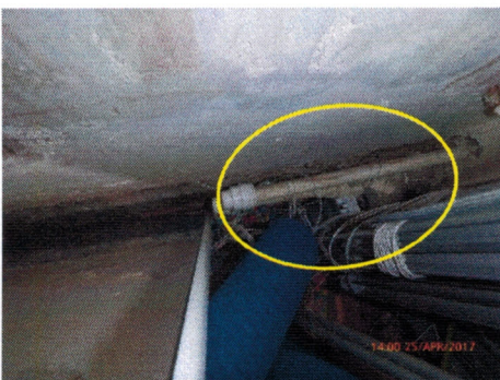
Photo 17: Deadend in Century house 1st floor store cupboard
